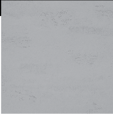
MOA-##-S | Pitted Surface
